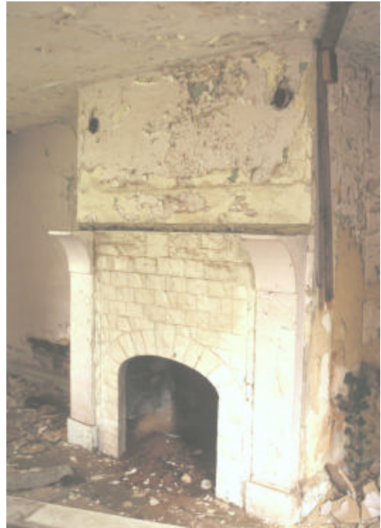
Figure 25. Remodeled fireplace on the first floor of the original log portion of the Isaac and Margaret Sharp house.
