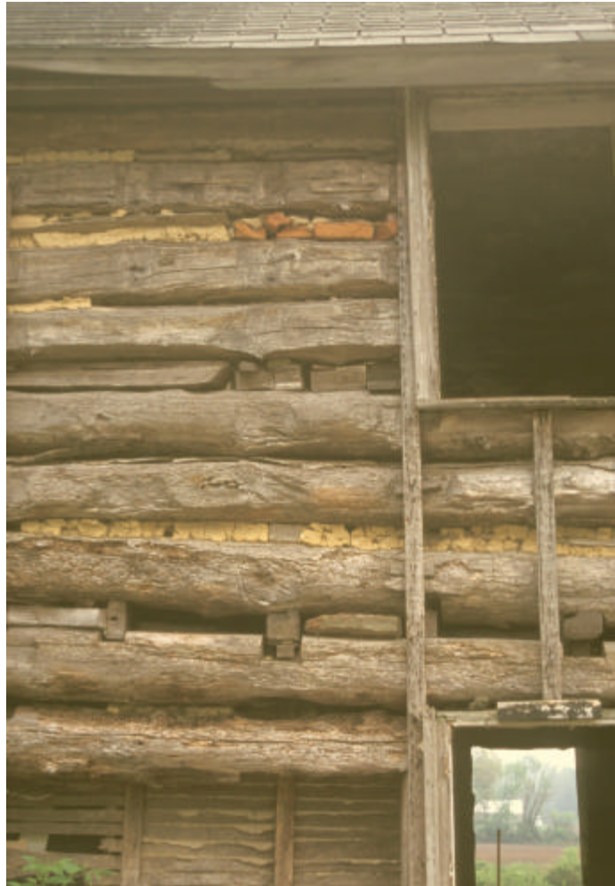
Figure 13. Detail of rear of Isaac and Margaret Sharp house. Illustrates several chinking materials including wood, mud, and later brick.
