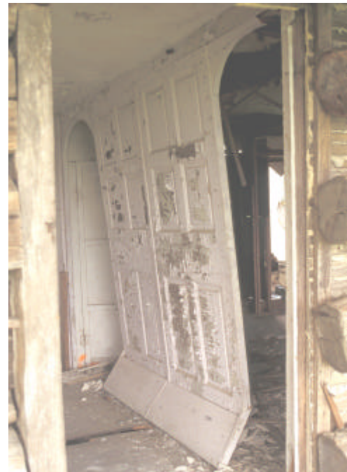
Figure 24. Nineteenth-century partition between the two first-floor rooms in the original log portion of the Isaac and Margaret Sharp house.
