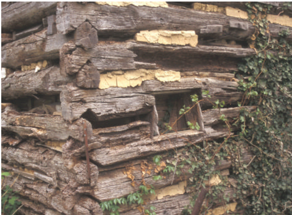
Figure 12. View of visible gable end of the Isaac and Margaret Sharp house. Alternating tiers and V-notch joinery are visible at the corner of the building.
