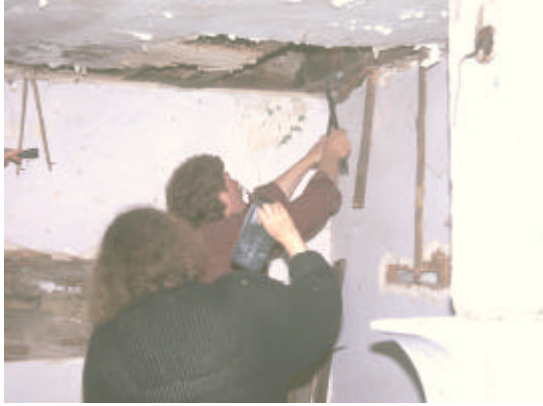
Figure 10. Bernard Herman and Gabrielle Lanier removing plaster and lath in an attempt to find evidence of a staircase leading from the first to the second floor of the Isaac and Margaret Sharp house.
