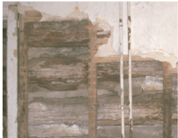
Figure 34. Detail of the interior gable-end wall in the parlor of the Isaac and Margaret Sharp house. Shows white-washed logs and bark.
