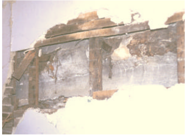
Figure 35. Rear wall in the common room of the Isaac and Margaret Sharp house. The undulating plaster coat that is visible in this photograph represented a second stage of interior finish.
