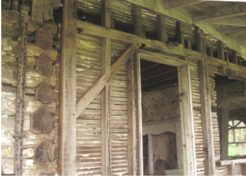
Figure 23. Detail of area where the nineteenth-century frame addition was added to the original Isaac and Margaret Sharp house. Note braced-frame construction.
