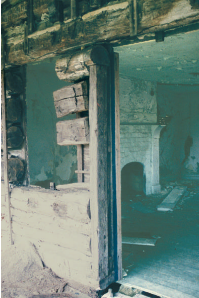
Figure 15. Front door opening at Isaac and Margaret Sharp house. The vertical wooden member is pegged into the surrounding logs.
