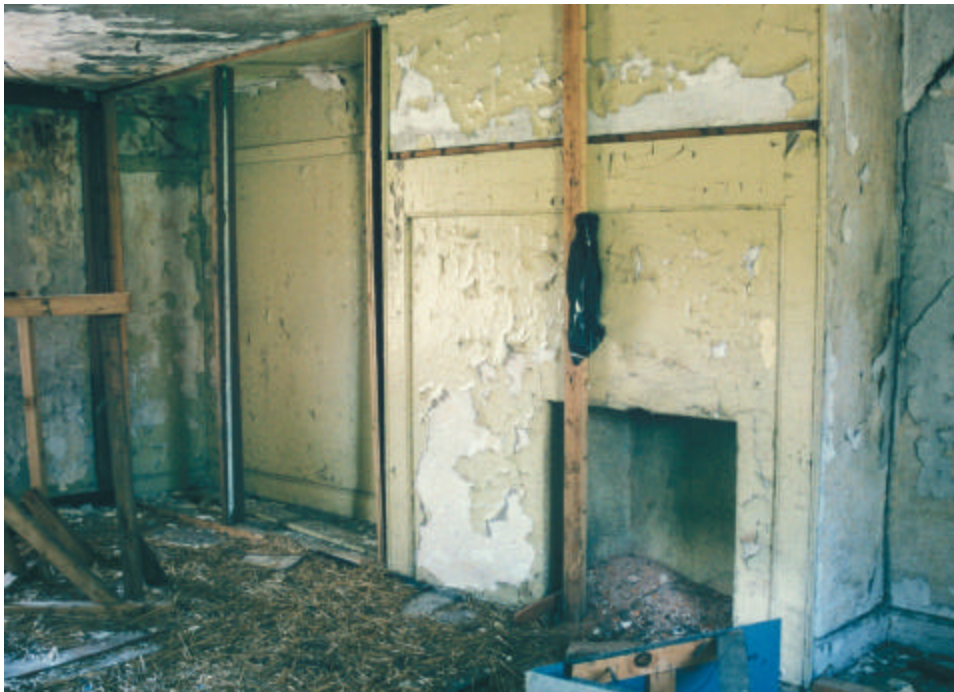
Figure 21. Fireplace on the second floor of the Isaac and Margaret Sharp house. This fireplace may date to 1782, when the house was originally constructed.
