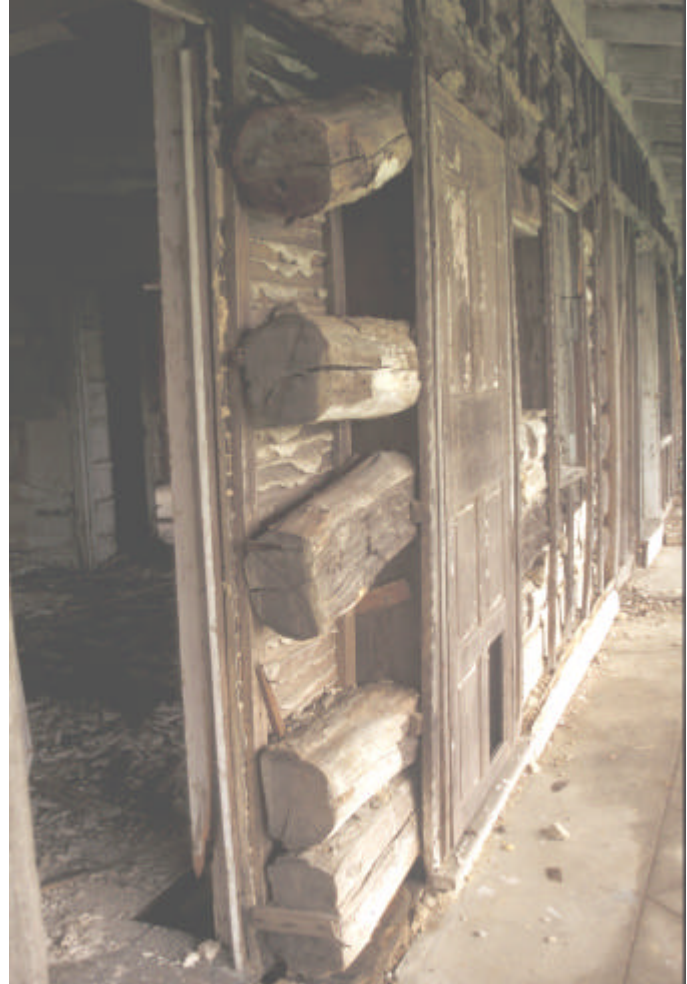
Figure 11. Detail from façade of the Isaac and Margaret Sharp house. Shows both the round and the very roughly hewed logs used to construct the building.
