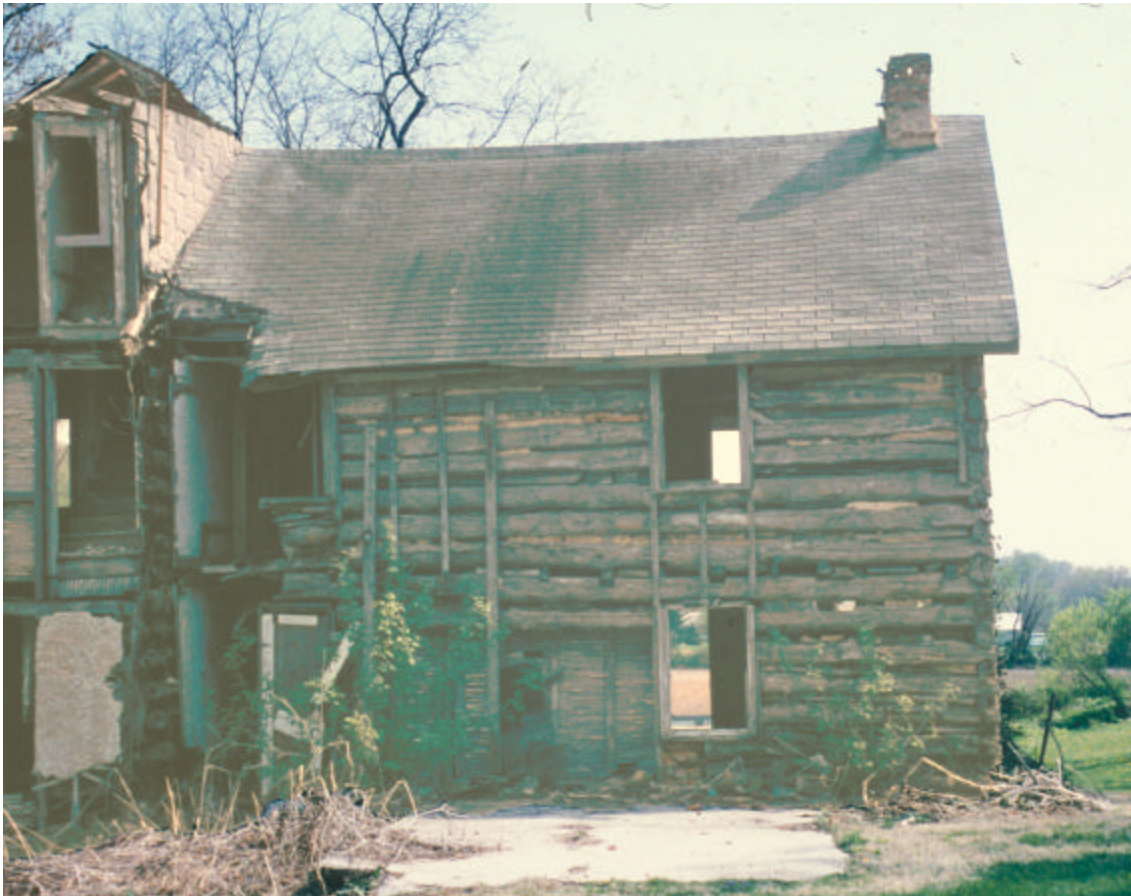
Figure 28. View of the rear of the Isaac and Margaret Sharp house. In order to facilitate the application of stucco, furring strips were applied over the log portion of the house.
