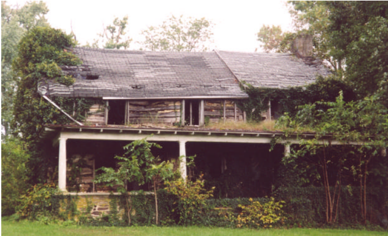
Figure 1. Isaac and Margaret Sharp House (New Garden Township, Chester County, Pennsylvania, 1782) as it appeared in September 2003. The vine-covered frame structure (to the right) and the front porch are later additions.
