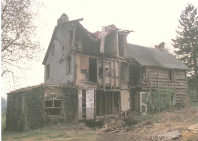
Figure 29. View of the rear of the Isaac and Margaret Sharp house and its subsequent additions. The room that occupies the third floor (or garret) of the frame addition was designed to be Thomas Eakin's studio.
