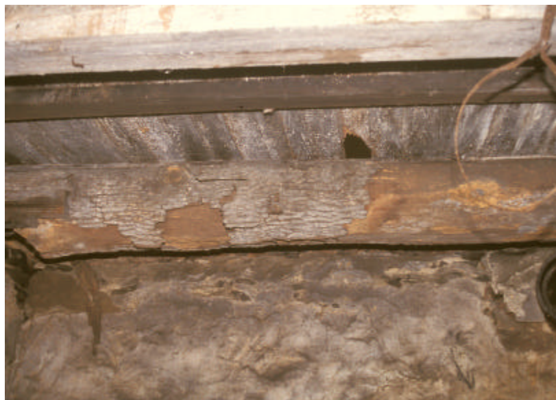
Figure 19. Surviving original joist in the cellar of the Isaac and Margaret Sharp house.
